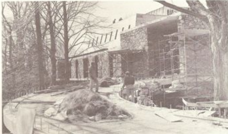
Construction is more than 50 percent complete on the major addition to the library.
